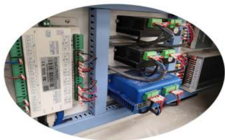
Control cabinet with RD laserword
